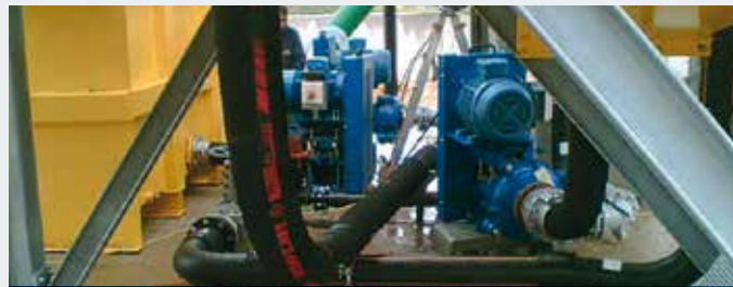
Underflow screening machine, cyclones and pumps deployed for sand classification , for every 100 m 3 /h Pump 1: for sand 0.5 – 2 mm, 50 t/h, separating cut approx. 0.063 mm Pump 2: for sand 0 – 0.5 mm, 30 – 40 t/h, separating cut at approx. 0.063 mm
